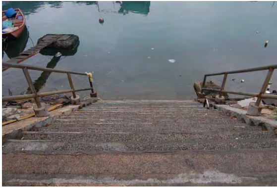
Figure 4.47: Stairwell to Polluted Water in Lei Yue Mun Typhoon Shelter
